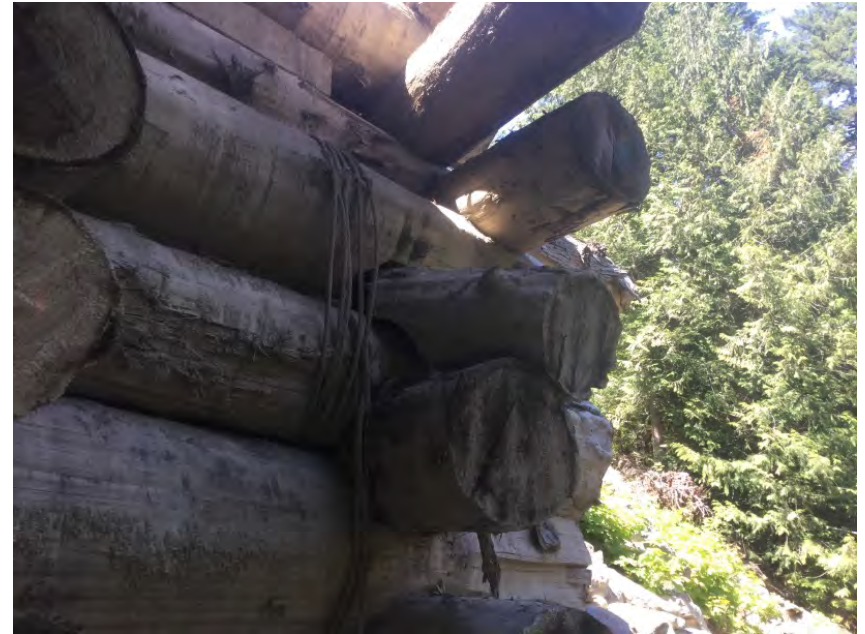
Broken tieback upstream right abutment
